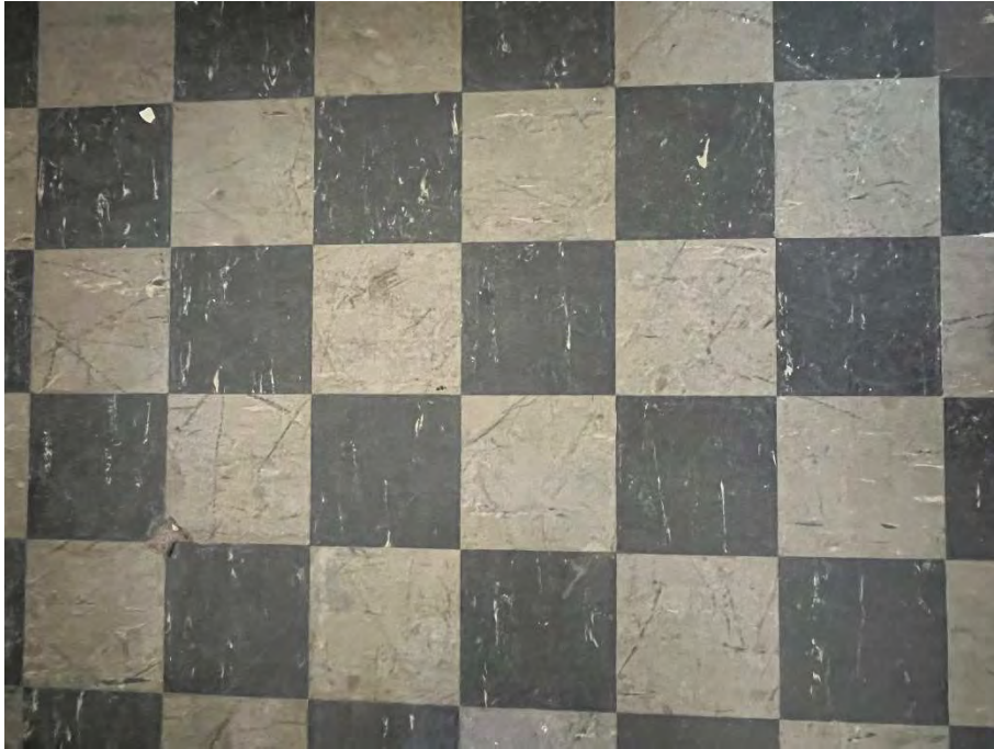
Photo of existing / original vinyl composition tile floor. This is an example of a floor finish material that may contain asbestos. It is also possible that the flooring mastic may contain asbestos as well.
