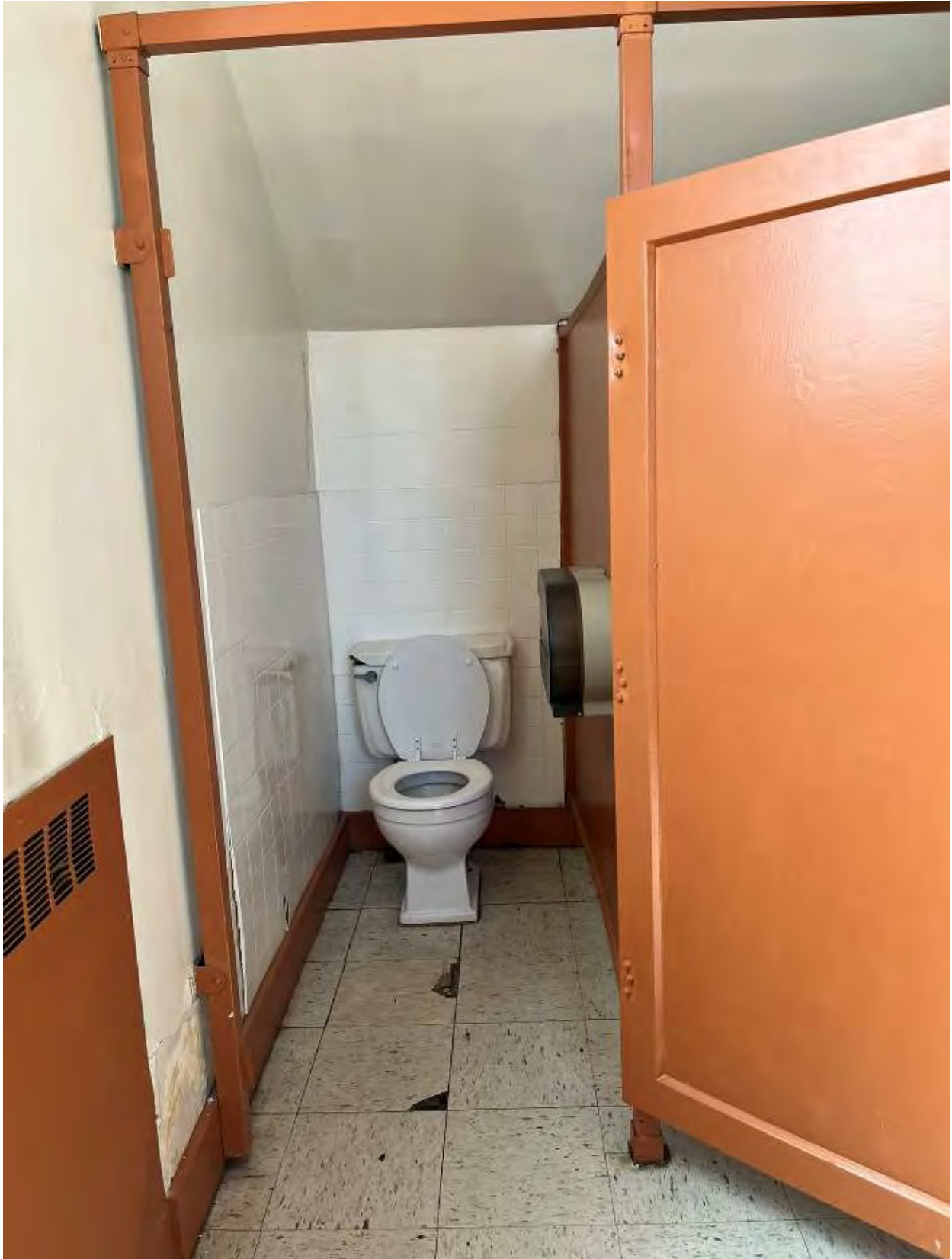
Photo of deteriorating flooring in bathroom, which appears to be asbestos containing tile / mastic.
