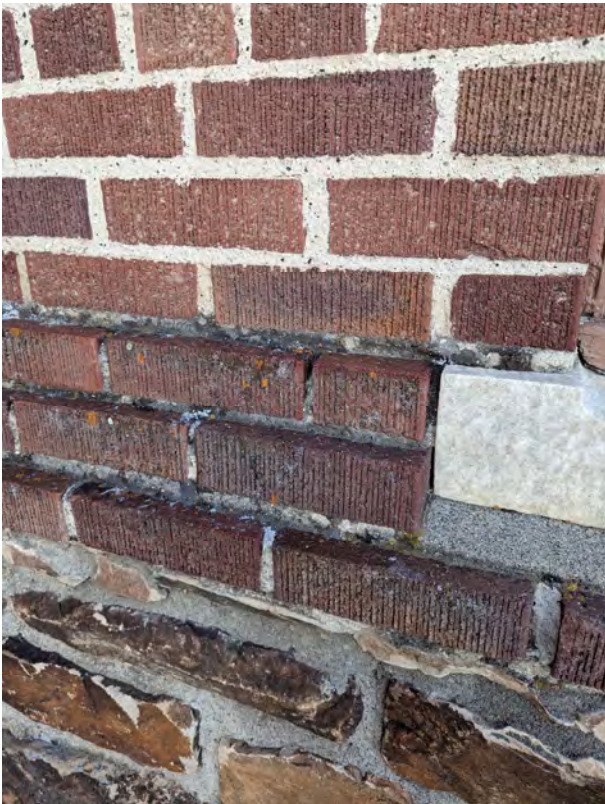
View of deteriorating grout (Item S6).
