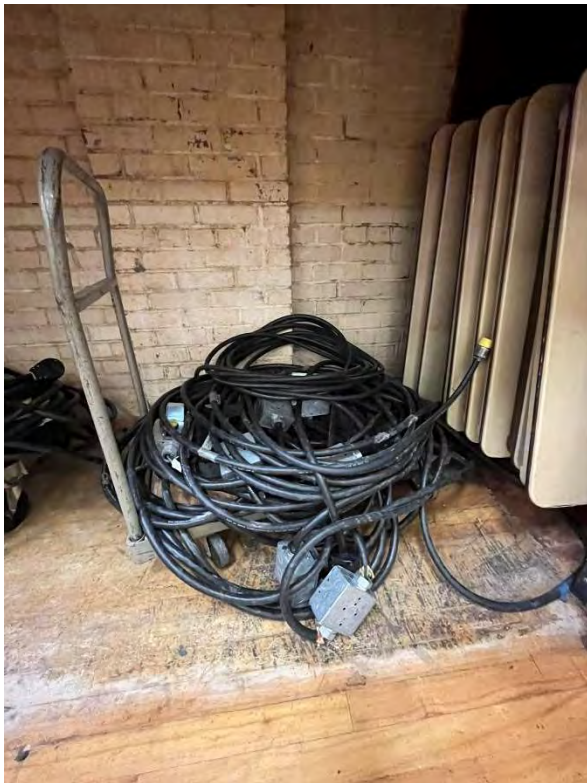
Photo of cable and floor boxes.
