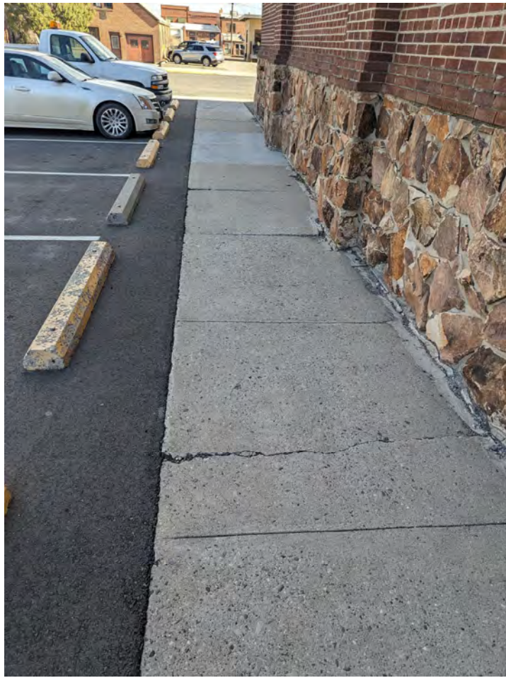
View of uneven sidewalk and spalling (item S7).
