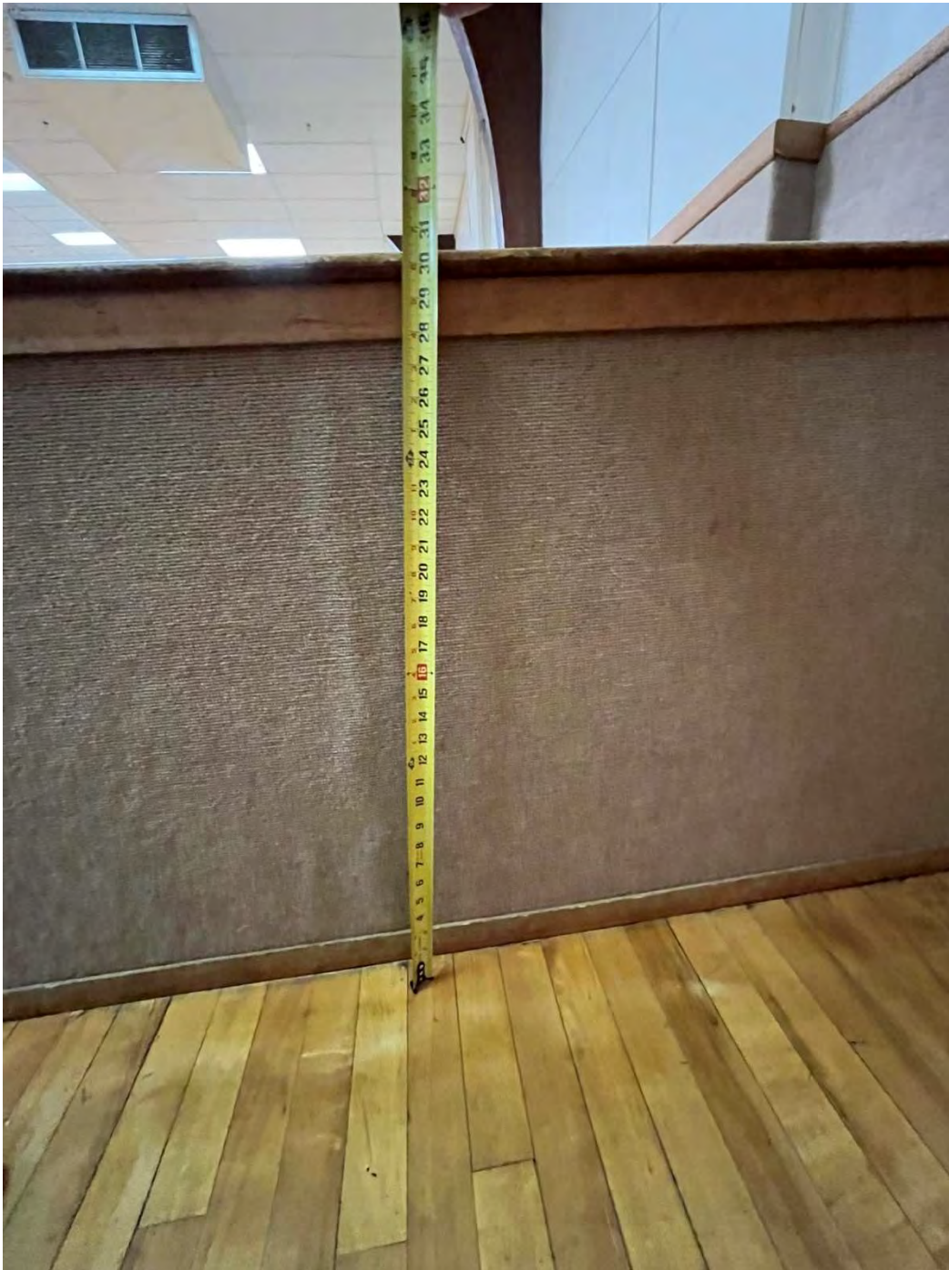
Photo of non-complaint height on wing walls at top of stairs. This requires a 42" top rail with a 36" high handrail.
