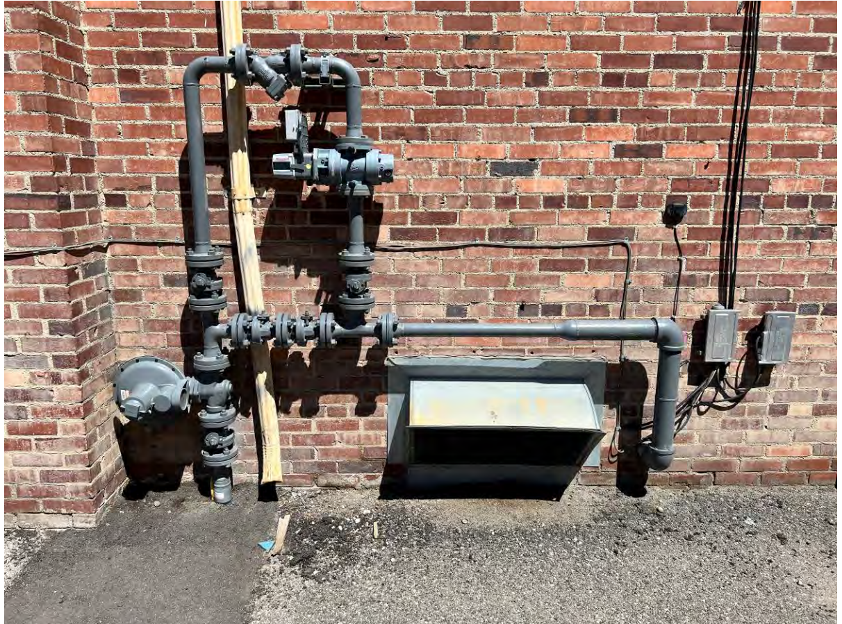
Natural gas regulator with gas line to boiler room. Combustion air hood near ground level.
