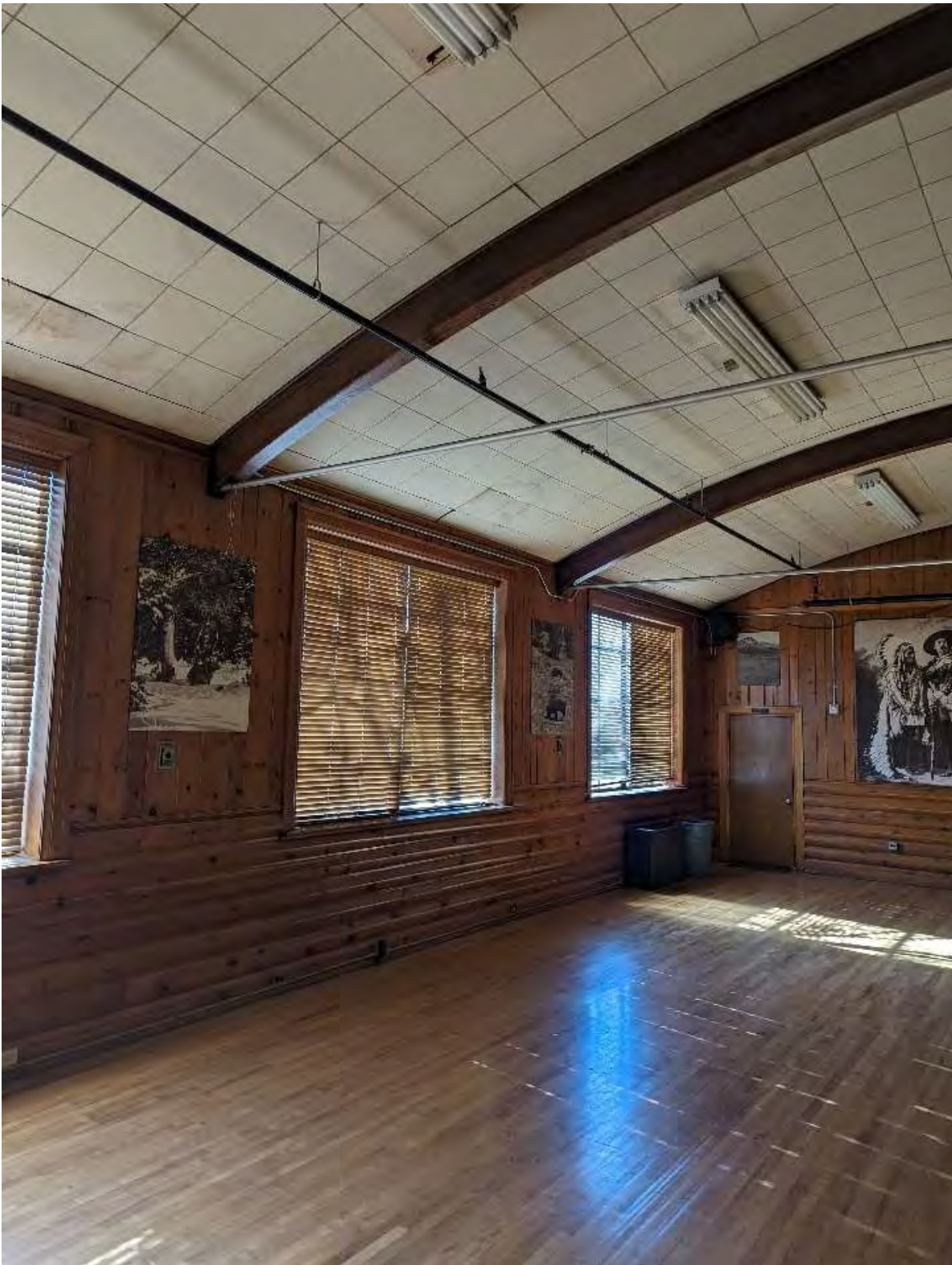
Photo of existing ceiling in club room. Stained and misshaped ceiling tiles are an indication of water damage and infiltration.
