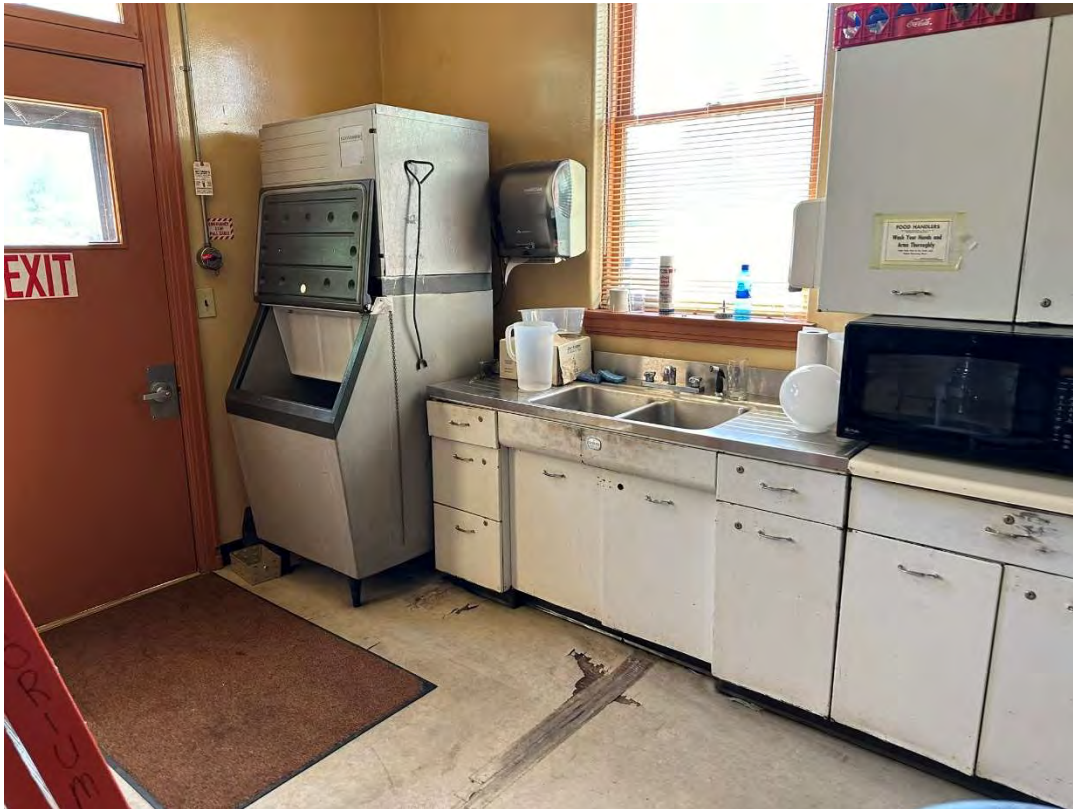
Photo of kitchen floor at sink. Note the floor finish is showing signs of water and other damage.
