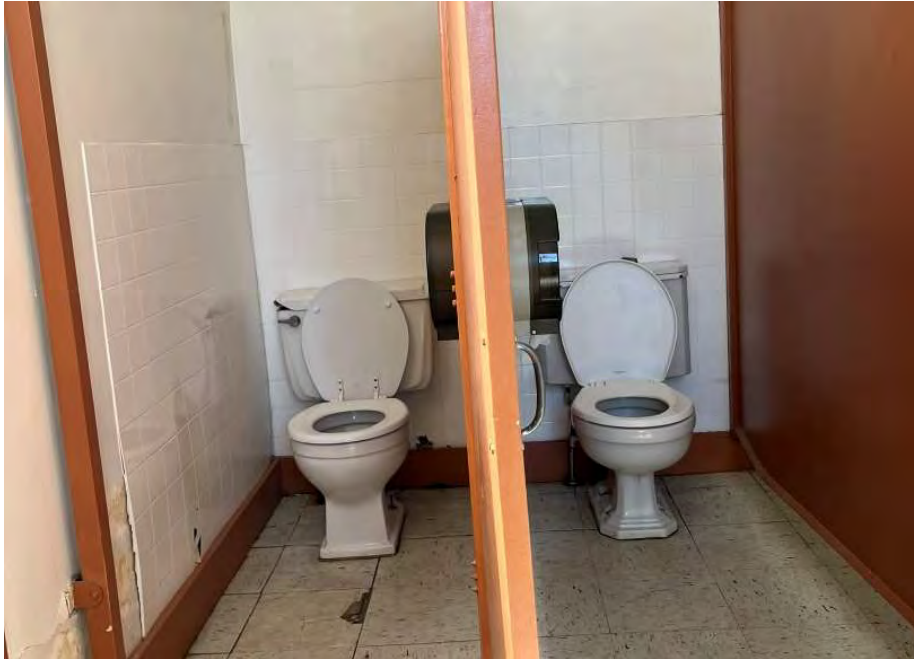
Photo of non-ADA compliant bathroom stalls. See ADA diagrams attached herein.
