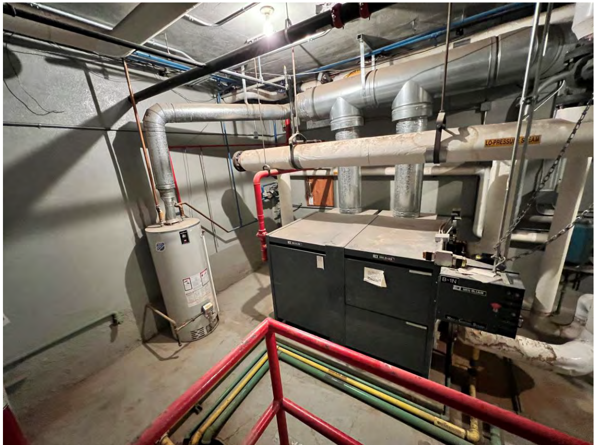
Boiler, venting and water heater.
