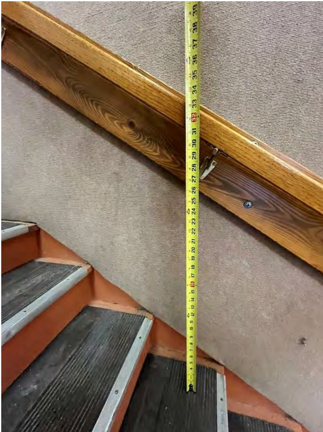
Photo of incorrect height of handrails at stairs. This is required to be at 36" above the stair nosing.
