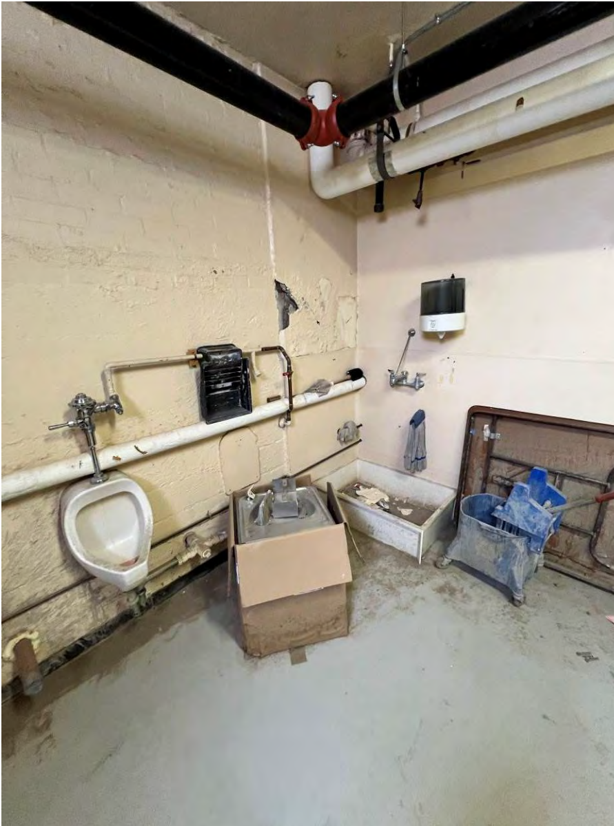
Odd- Urinal in basement mechanical room
