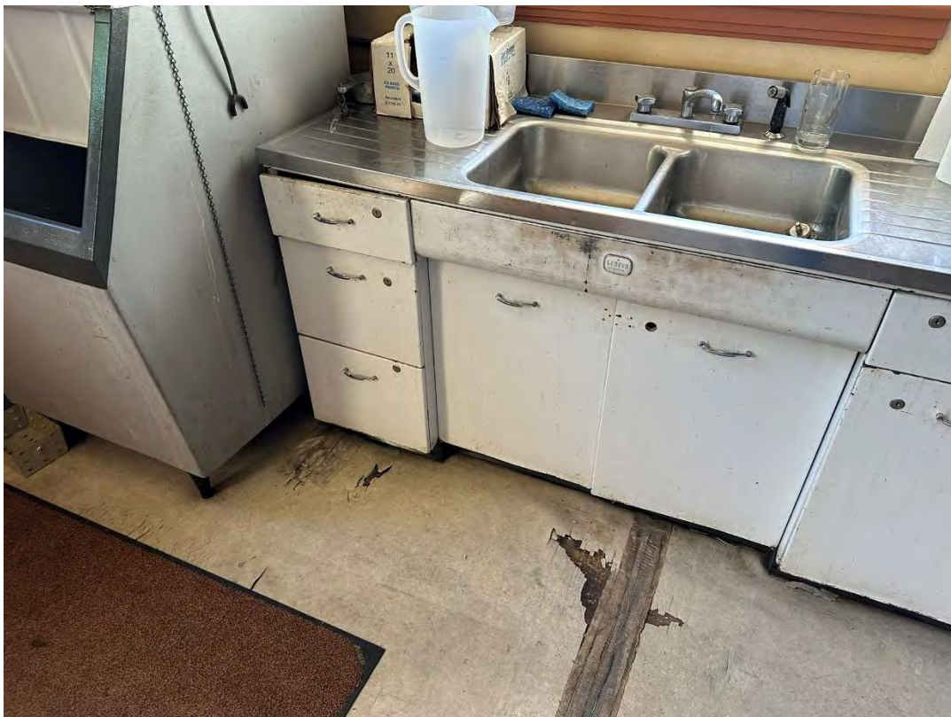
Enlarged photograph of damage to the kitchen flooring. Note the areas where the linoleum is missing exposing the sub-floor below as well as areas where the flooring material has bubbled due to water intrusion and other damage. This location also presents a tripping hazard.
