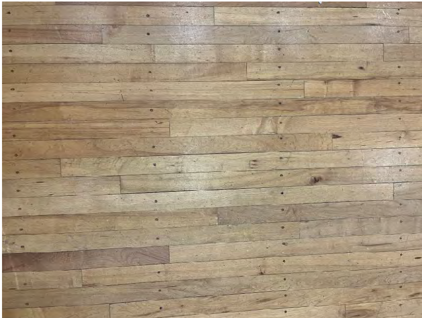
Photo of exposed fasteners in the main auditorium floor.
