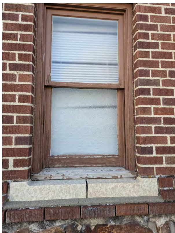
View of deteriorating grout (Item S6).
