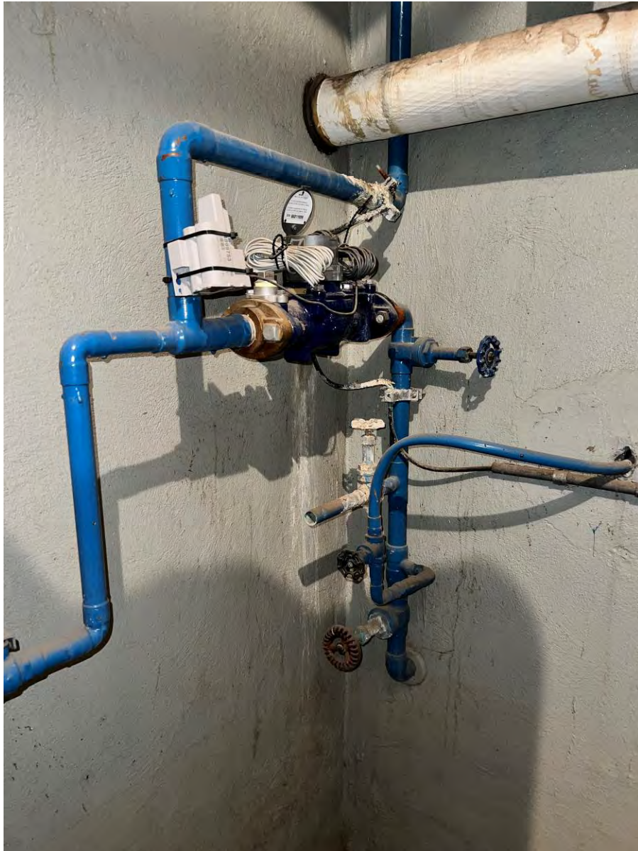
Water Service into building
