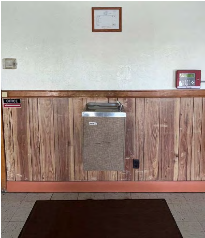
Photo of non-ADA compliant drinking fountain. See ADA diagrams attached herein.
