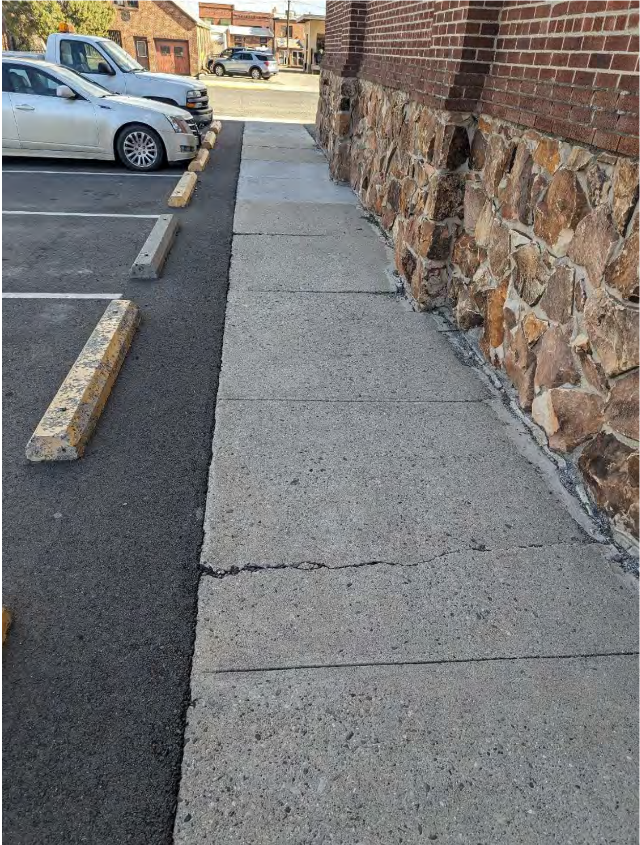
Photo of spalling and uneven concrete sidewalk.
