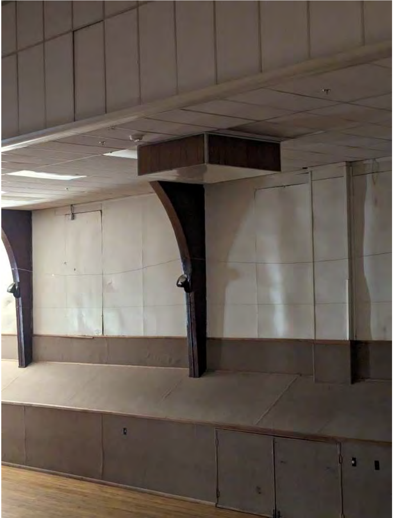
Photo of existing wall paneling in auditorium with deteriorating paneling.
