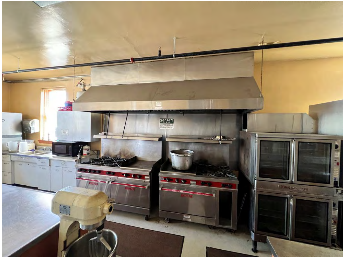
Kitchen equipment under the hood – no hood over oven
